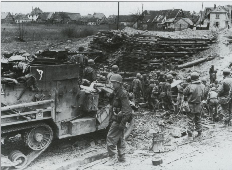
Engineers of the 125th Engineer Battalion, 14th Armored Division complete work on the pilings for a bridge over the Seltzbach river near Niederroedern on 18 March 1945, with a M3A1 half-track from the unit in the foreground.
